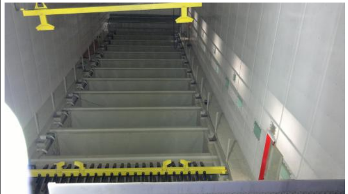
Chemical pre-treatment in the housing
